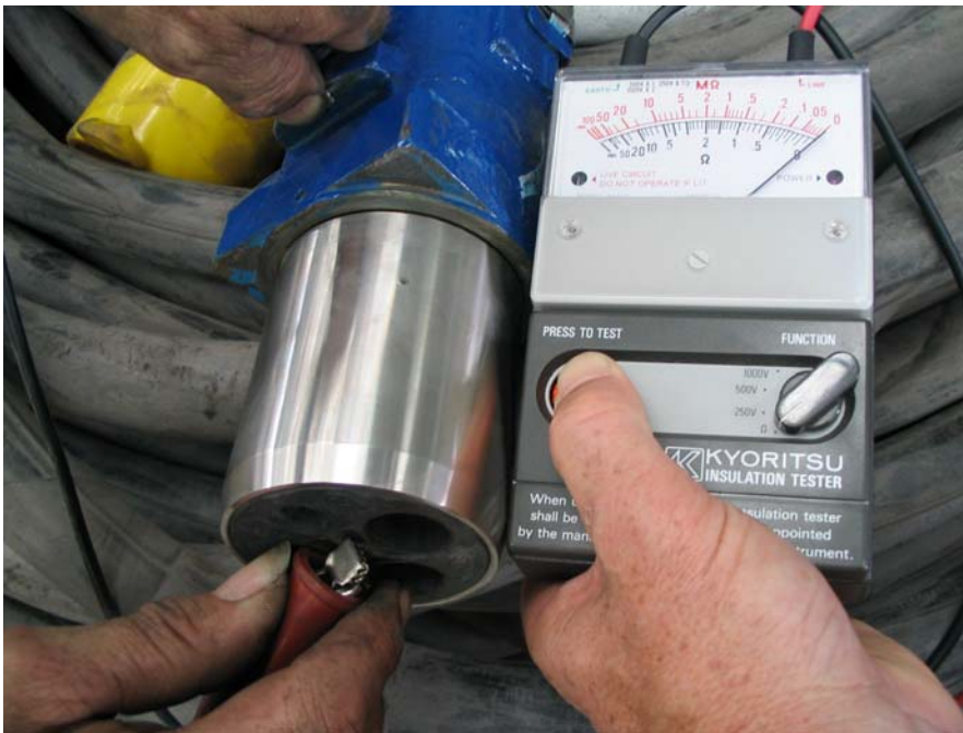
Figure 24: Earth continuity test from phase barrier to plug body for a typical 150 Amp restrained plug
