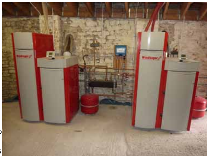
Example of a small scale biomass heating system
