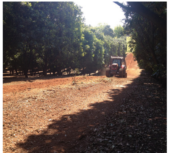
A row of trees has been removed and the ground is being shaped for an inter-row drain.
