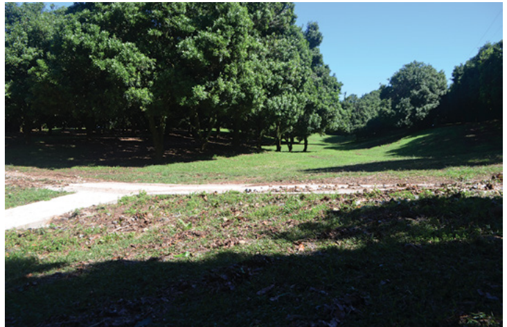
Some concrete was used to allow an access road to cross this grassed watercourse. The trafficked pathway had been scouring out, needing more than grass cover to protect it.
