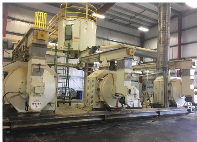
Figure 2: Pellet mills at the Altus Renewables facility in Maryborough, Queensland
