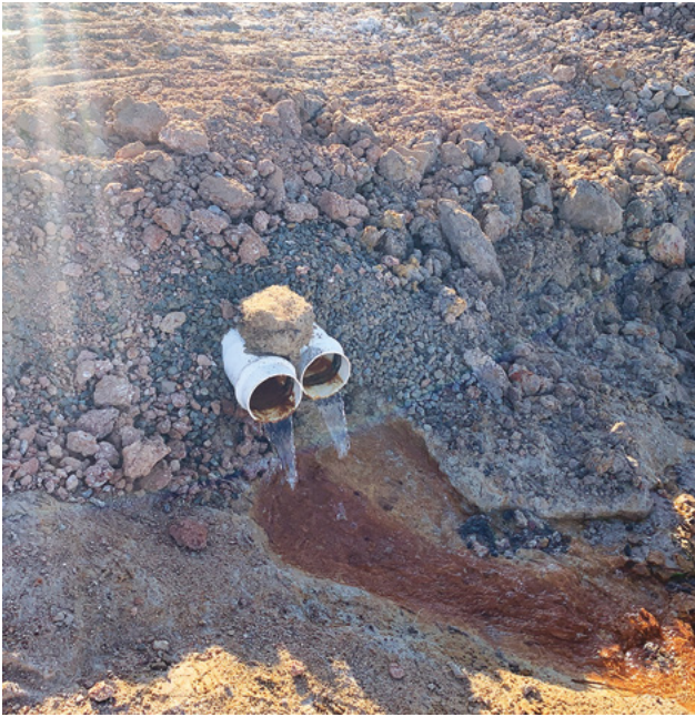
Figure 48. This outlet for a network of sub-surface drains brings water into a storage dam and provides a convenient water sampling point for nutrient monitoring.
