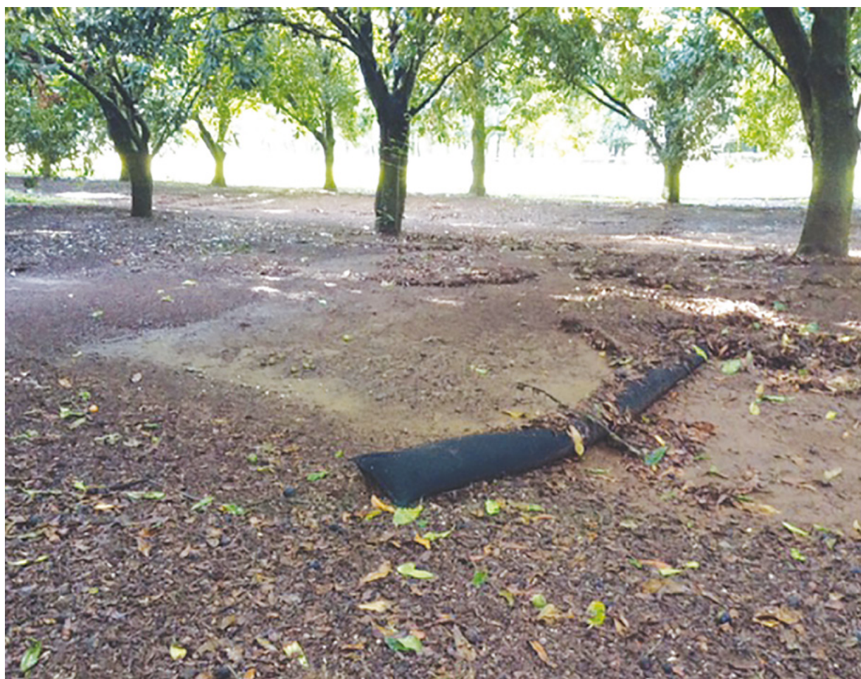
Figure 40. Once filled with sediment, the check structure is no longer effective.
