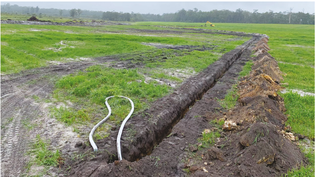
Figure 50. This drain will prevent the surface soil in the lowest areas from being waterlogged for long periods.
