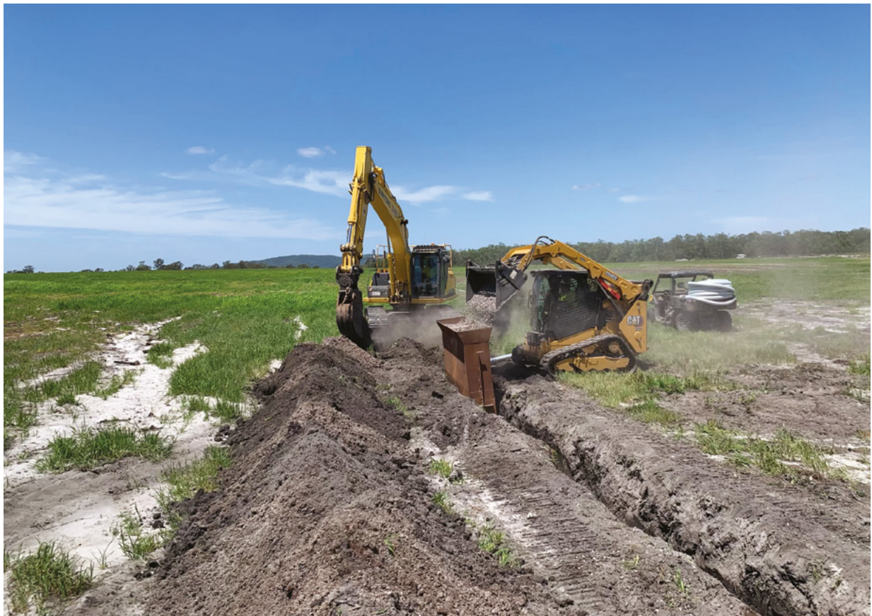
Figure 47. A sub-surface drain being constructed; an excavator opens the trench, ag-pipe is laid into the trench, backfilled with gravel via a slot-shaped funnel that can be slid along inside the trench.
