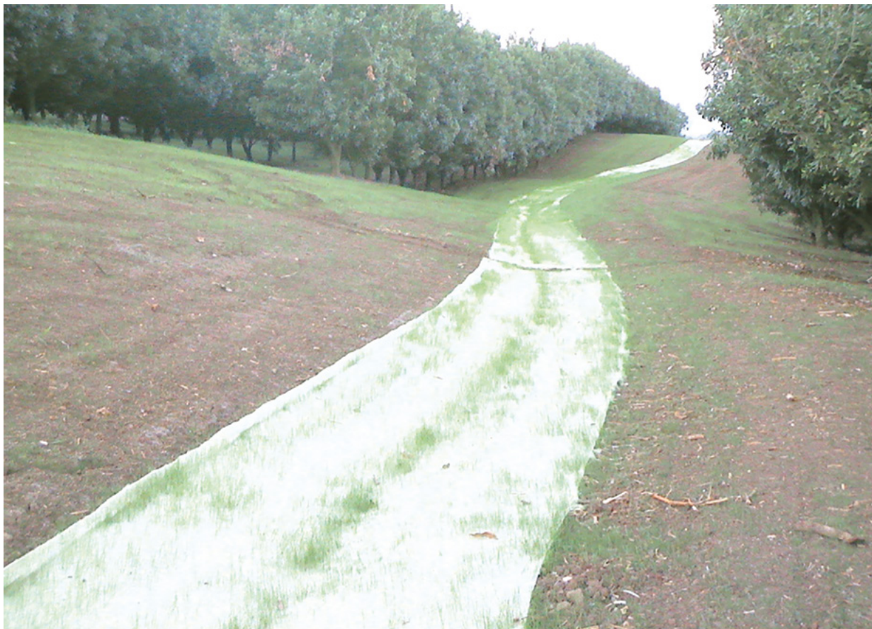
Figure 38. A recently constructed diversion bank where jute erosion control matting has been laid in the flow path and a ryegrass cover crop is emerging.
