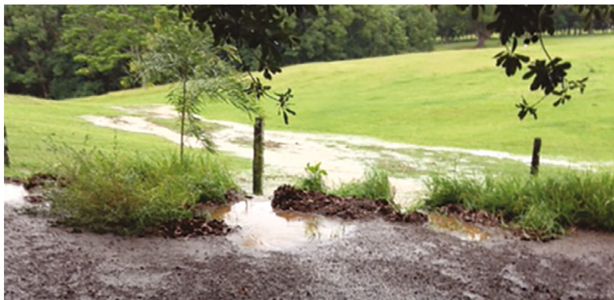
Figure 8. A sediment trap reduces the amount of soil moving into the neighbour's paddock.
