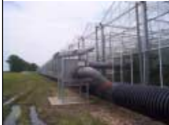
Top: Electricity generators are installed as part of a greenhouse complex for co-generation of power and heat. Middle: Carbon dioxide gas is extracted from the hot water boiler for use in the greenhouse. Bottom: Waste carbon dioxide gas is pumped from a nearby factory.
