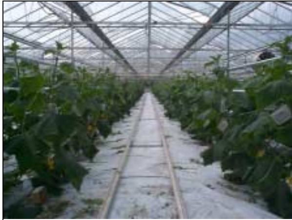
Piped hot water is preferred method of greenhouse heating and is standard practice. The pipes can also be used as rails to improve labour efficiency.
