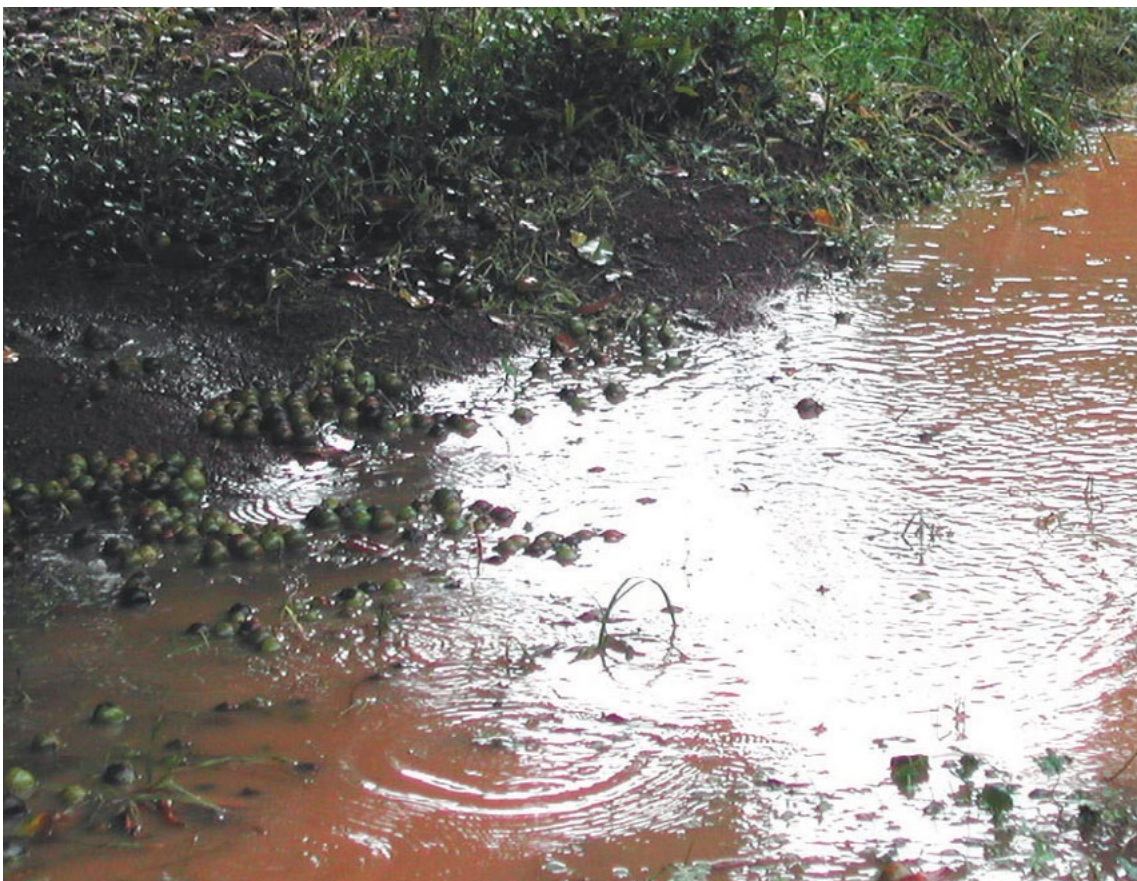
Figure 12. Nuts in drains and muddy run-off water are signs of active soil erosion.
