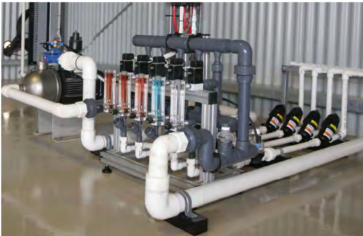
Figure 5. A fully automated multi-tank Venturi injection system.
