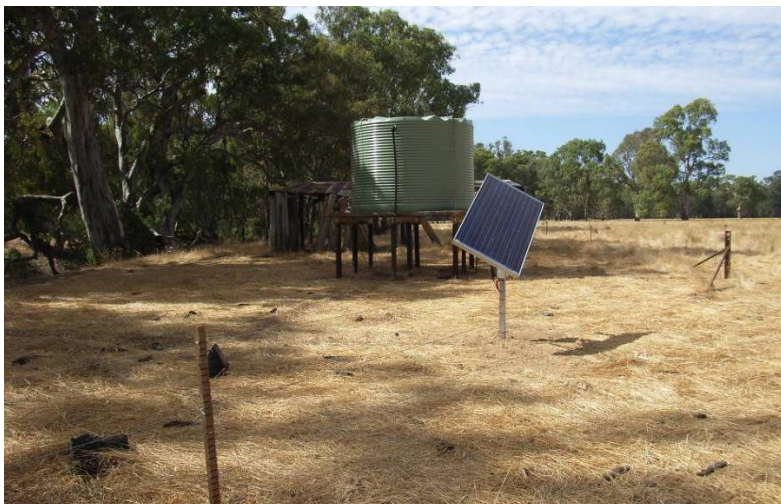
Image 4: The 150W solar panel powers a submersible pump which provides water to the header tank. The troughs are gravity fed from the tank. Even relatively small systems like this one are expensive to install. The costs have to be justifiable in terms of the quality and size of the area being protected.
