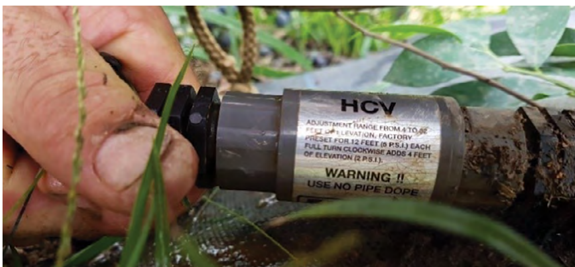
Figure 19. Check valves can reduce the drainage from mains to the lowest dripper. Photo: Robert Hoogers.
