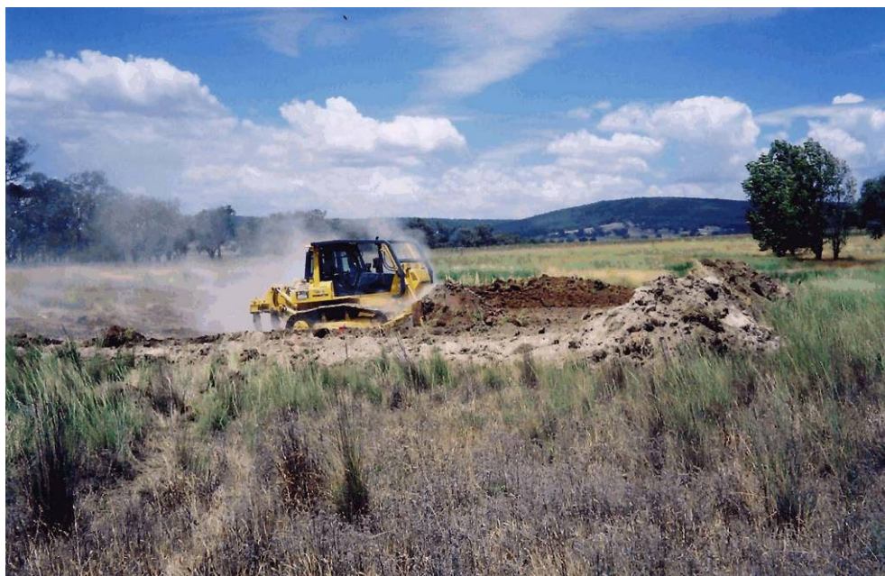
Image 37: Work commences on Ian McColl's constructed wetland (February 2003). Essentially a modified farm dam, the wetland incorporates an island and was built to provide areas with differing water depths. A 100mm spillway by-pass pipe was also installed through the dam wall which carries the base flows, keeping the spillway dry.
