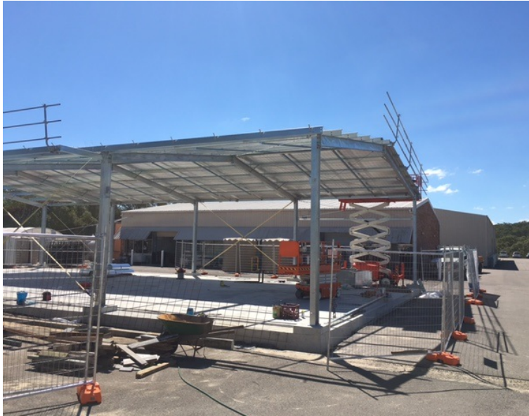
New nurse tank area at PSFI next to the hatchery and broodstock building
