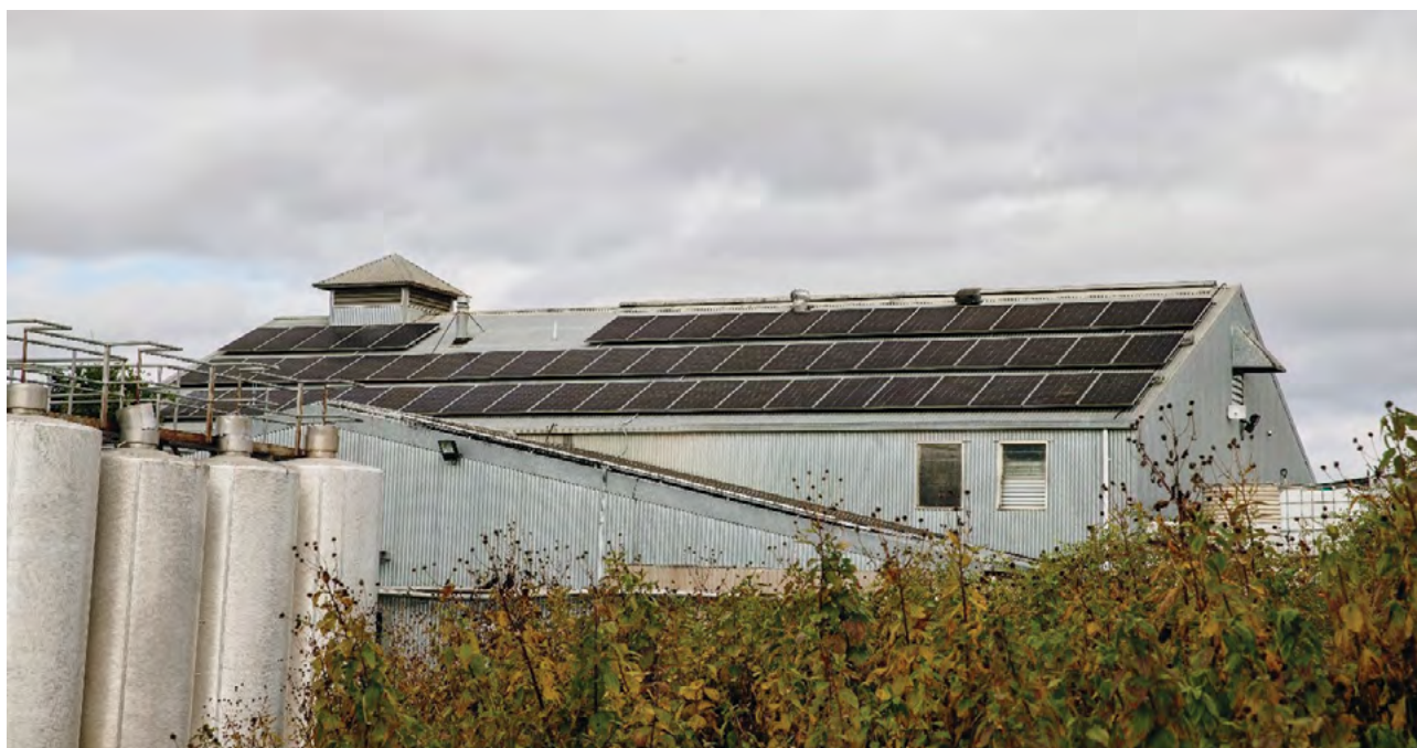
Figure 15. Solar panels on the winery roof at Lowe Wines, Mudgee NSW.
