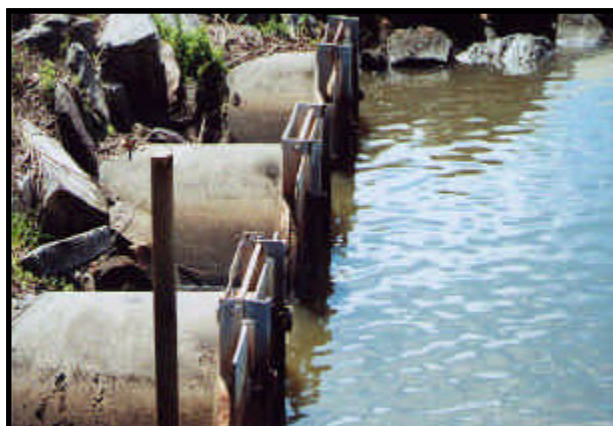
Fig 2. Floodgates on the lower Clarence. (Picture by Christina Collins, 2002)
