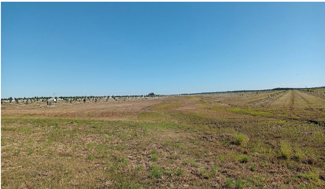
Figure 32. This newly formed grassed watercourse had scoured out, losing some soil from the centre. The surface has been smoothed and re-sown with grasses to stabilise the flow line.
