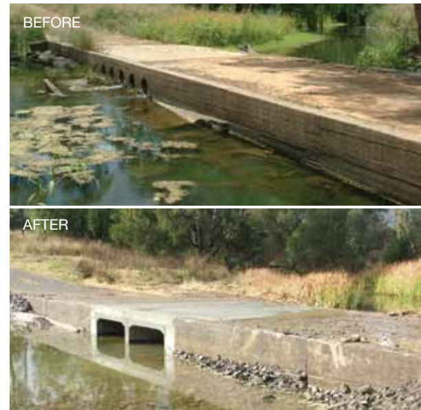
Over 5 km of upstream habitat in Halls Creek, a tributary of the Namoi River, was opened for fish passage following the remediation of this piped causeway with box culverts by Tamworth Regional Council. Funding assistance was provided by the Namoi Catchment Management Authority and the MDBA. (Images NSW DPI)
