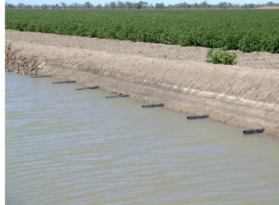
Permanent pipes through the bank (PTB) at Waverley, Wee Waa
