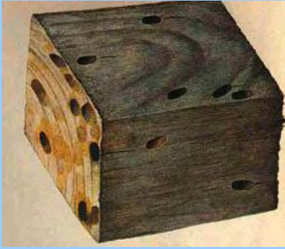
Above: Off-cut of timber exhibiting oval-shape exit holes caused by emerging adult beetles
