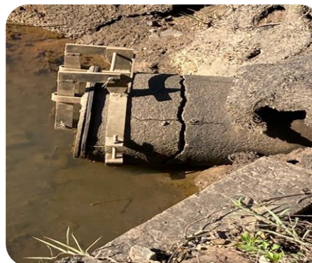
Figure 7: Showing cracked pipe and an outlet that cannot open due to siltation and collapsing concrete surrounds
