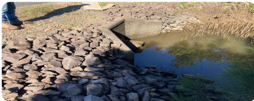
Figure 8: Showing a cracked pipe end (missing outlet) and mangrove encroachment
