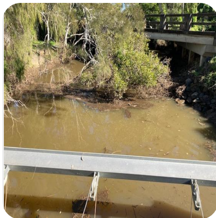
Figure 5: Drain constrained by the encroachment of vegetation
