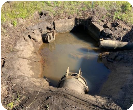
Figure 6: Showing cracked pipe and an outlet that cannot open due to siltation and collapsing concrete
