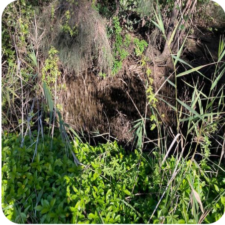
Figure 2: Drain blocked by vegetation
