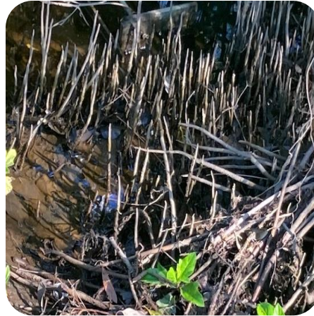
Figure 3 Drain blocked by mangrove pneumatophores
