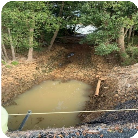
Figure 4: Drain constrained by the encroachment of spoil
