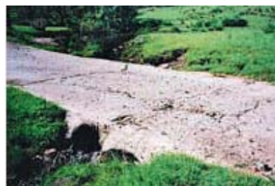
Barrier to fish passage on the Severn River (2004). A round narrow pipe restricts flow and prevents upstream migration of fish.
