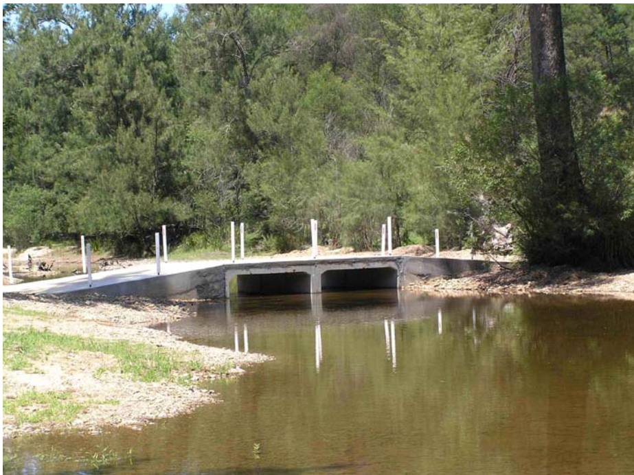
Figure 9. Quart Pot Road crossing a) prior to and b) after construction of a double box culvert.
