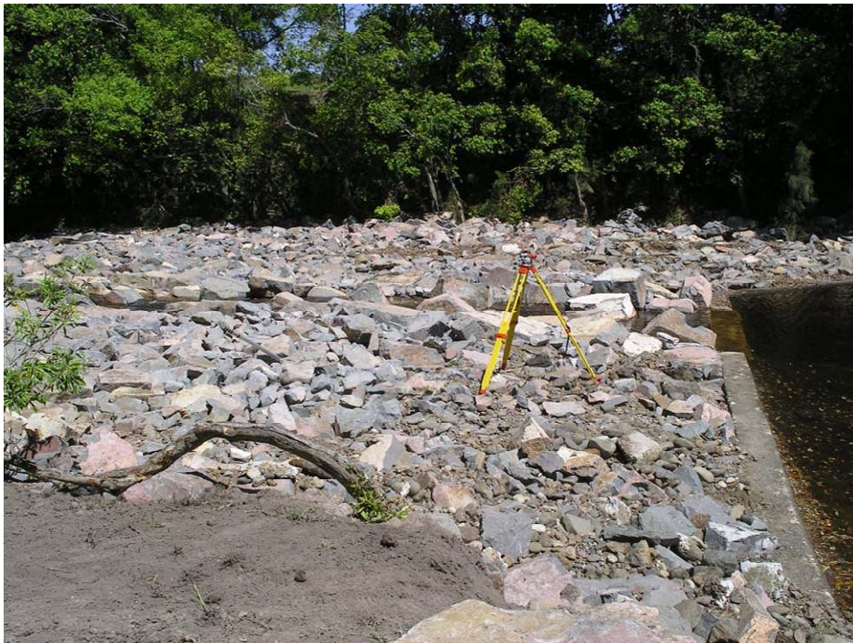
Figure 16. Stroud Weir a) prior to fishway construction and b) following fishway construction.
