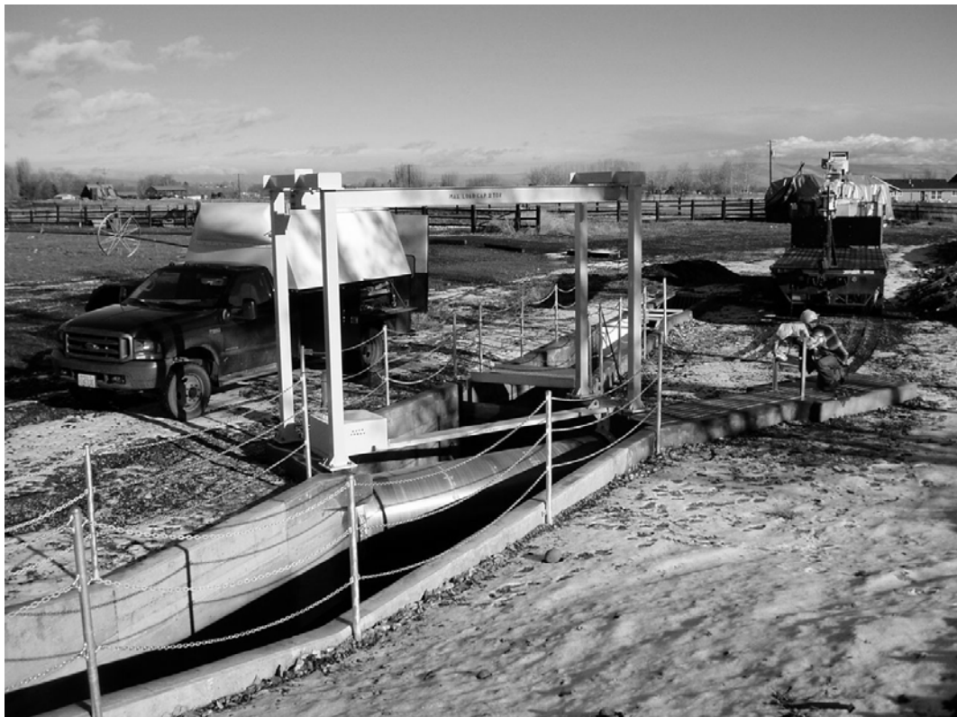
Figure 6.2. An example of a rotating drum screen installed on Cowiche Creek, Washington State USA. (Photo courtesy of the Washington Department of Fish and Wildlife).
