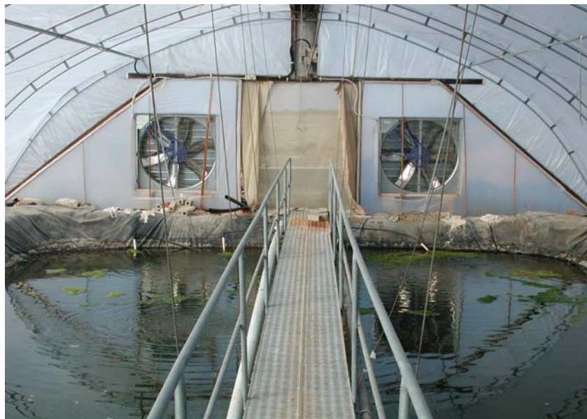
Figure 2. Air extraction fans (Munters TM EM50) installed in large polytunnel at CPISARC.
