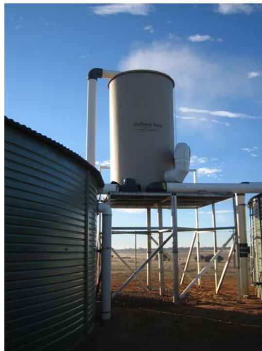
Figure 5. Packed column degasser installed to reduce dissolved carbon dioxide content of SIS groundwater used at WISAC.
