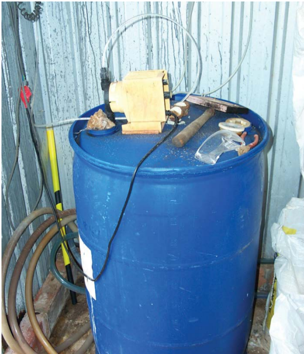
Figure 5: Automatic acid injection to adjust pH
