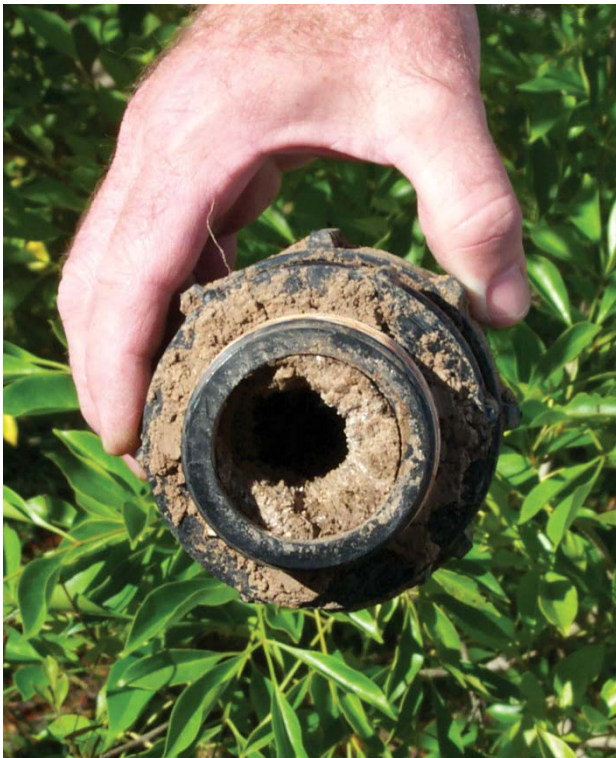
Figure 4. Lime build-up in pipes and equipment affects their performance.
