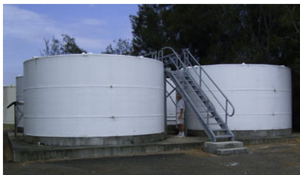
Fibreglass seawater storage tanks
