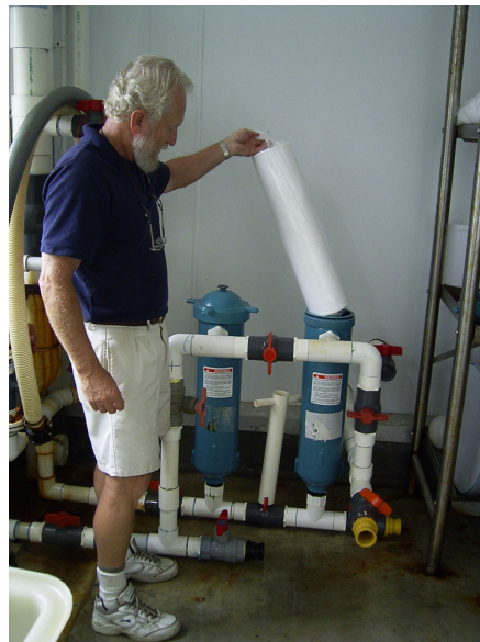
Hatchery seawater filters
