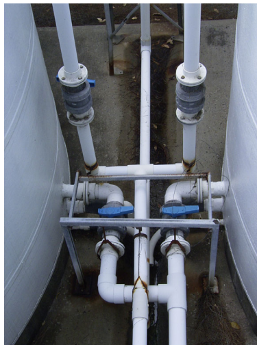
Water storage tank plumbing
