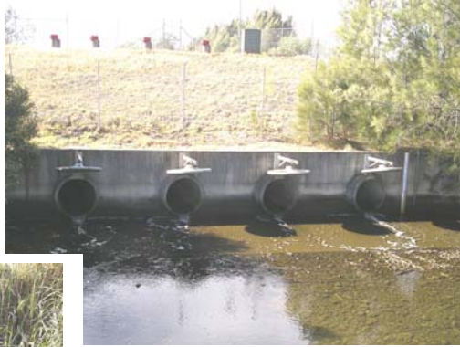
Photo 3: Floodgate – Kelso Creek, Lower Georges River subcatchment.
