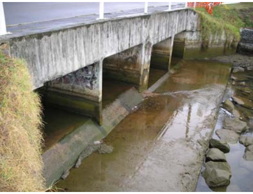
Photo 1: Road Culvert with raised invert, Gwawley Creek, Lower Georges River subcatchment.
