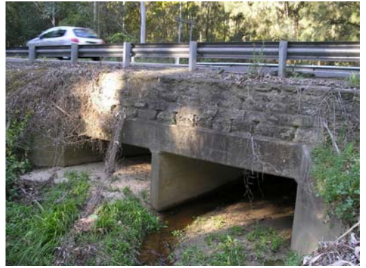
Photo 10: Partially silted road culvert, Little Blue Gum Creek, Middle Harbour / Lane Cove River subcatchment.
