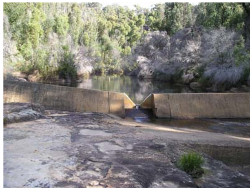
Photo 6: River Gauge Station, Stokes Creek, Upper Georges River subcatchment.
