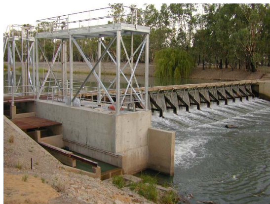
Figure 3. Balranald Weir showing a) the original submerged orifice fishway and b) the retrofitted Deelder fishlock.
