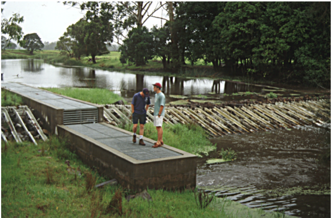
Figure 6. The new vertical slot Buladelah fishway.
