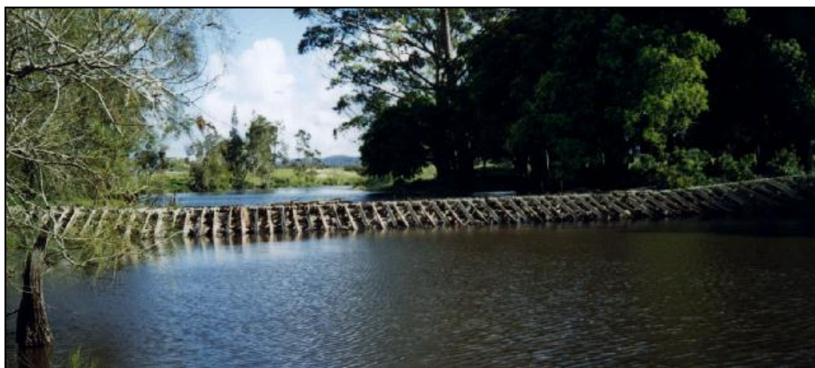
Figure 2. The Buladelah Weir located on the Crawford River about 75 m upstream from its junction with the Myall River, Buladelah, NSW, Australia.
