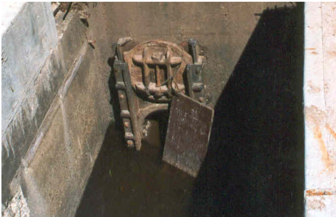
Figure 5. Exit pipe of original Buladelah Fishway. The pipe was 3 m long and had an internal diameter of 300 mm.
