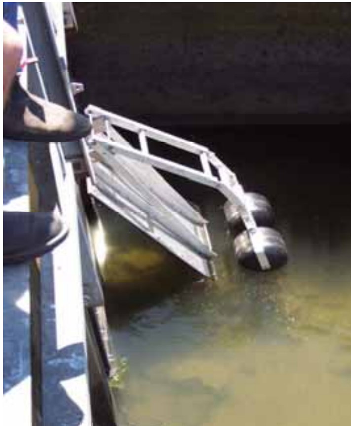
Figure A5.6. Tide-actuated floodgate at Greenways Creek in the Hunter catchment.
