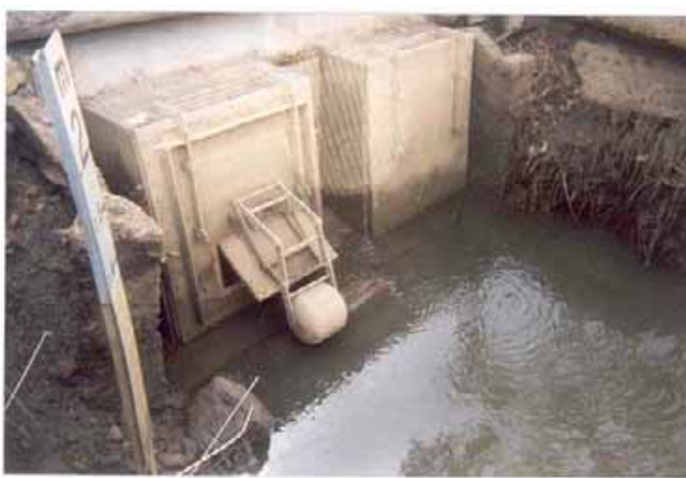
Figure A5.5. Tide-actuated floodgate at Fernbank Creek.
