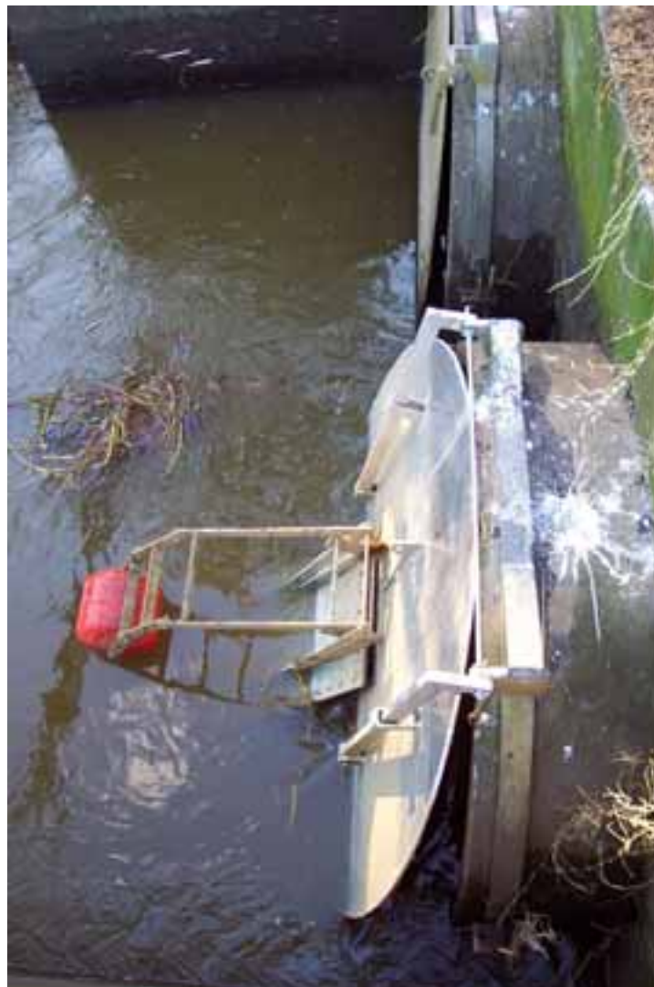
Figure A5.8. Differences in opening size during an outflow between a standard steel floodgate and an aluminium gate fitted with a tide-actuated internal gate.
