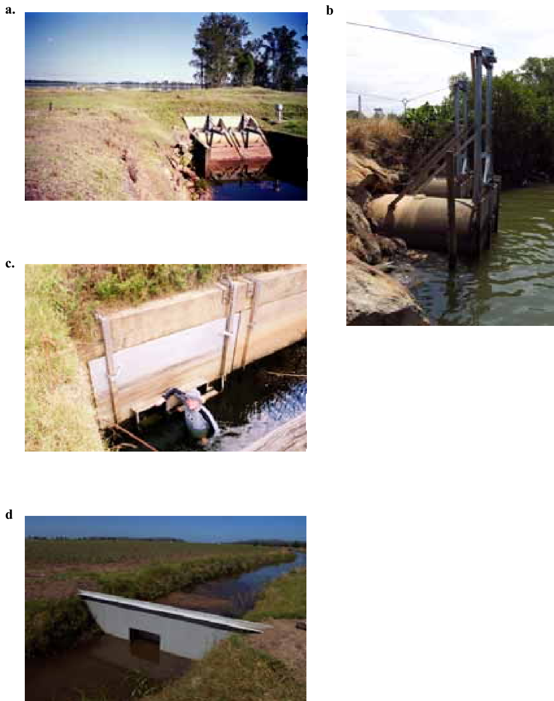
Figure 4.2. Floodgate openings and opening structures in the Clarence river floodplain; a. Wants Drain floodgates in open position, b. vertical liftgate on Marshes Drain, c. mini-sluicgate on Dennys Gully, and d. backwater retention structure in Dennys Gully. Note flooded grazing land on both sides of Wants Drain.
