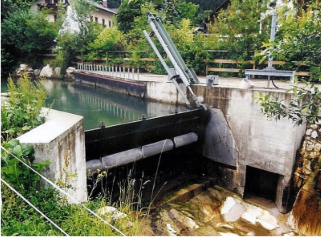
Figure 4.5. Example of a hydraulic tilt gate used to simulate overshoot flow (Photo Courtesy of Waterpower Engineering, UK).
