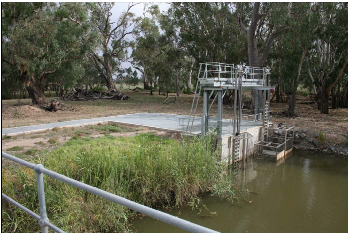
Figure 4.6. The Island Creek fishway exit with the WCSC separation cage fitted to one of the fishways upstream exit gates (on right). The WCSC can be mounted on either of the fishways exit gates using the same mounting brackets that support the trash racks (on left). Only the exit gate fitted with the WCSC is opened.
