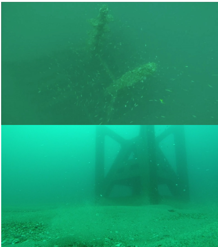
Figure 31 Inspections of the Sydney (upper image - 7 May 2015) and Shoalhaven (lower image - 18 May 2015) OARs following an intense east coast low that produced waves up to 15 m (Hmax)
