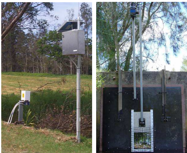
Image 36: left: smartgate system; right: motor and sensory equipment (W Glamore, UNSW)
