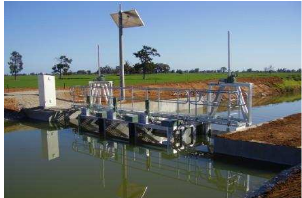
Image 55: fully automated and solar powered multi celled lay-flat gates (AWMA)
