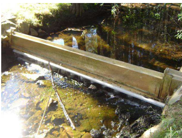
Image 48: rope fixed to tidal exclusion gate facilitates more efficient capacity for drainage by allowing greater opening span and periodicity during discharge
