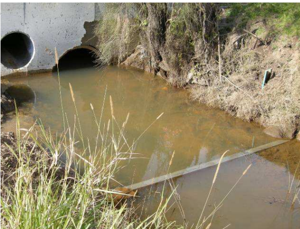
Image 46: sheet weir installed behind a culvert for ASS remediation in the Manning Valley
