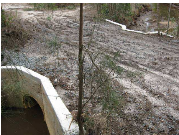
Image 6: concrete headwalls train flows through a culvert and provide protection against erosive processes (K Russell)
