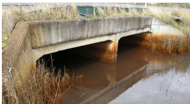
Image 3: concrete box culvert providing flow continuity of a channel under Nelson Bay Road
