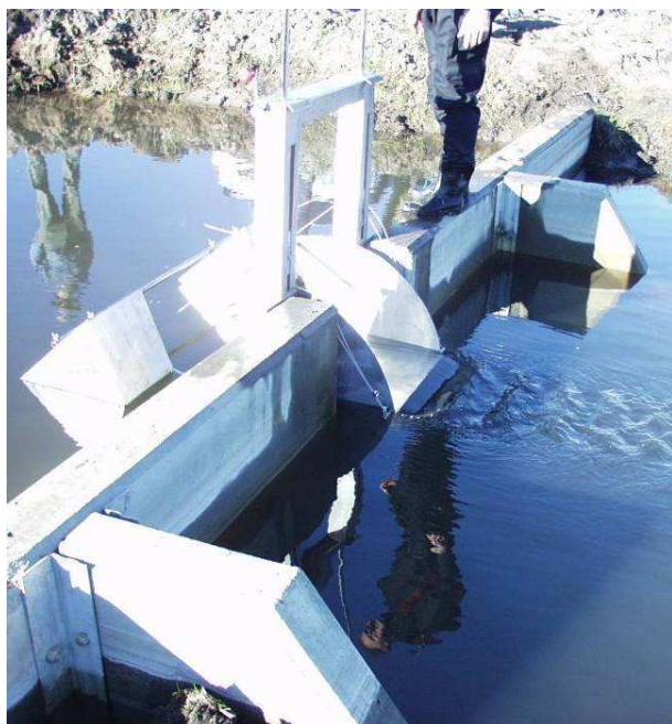
Image 59: water transfer through self tilting weir (W Glamore, UNSW Water Research Laboratory)
