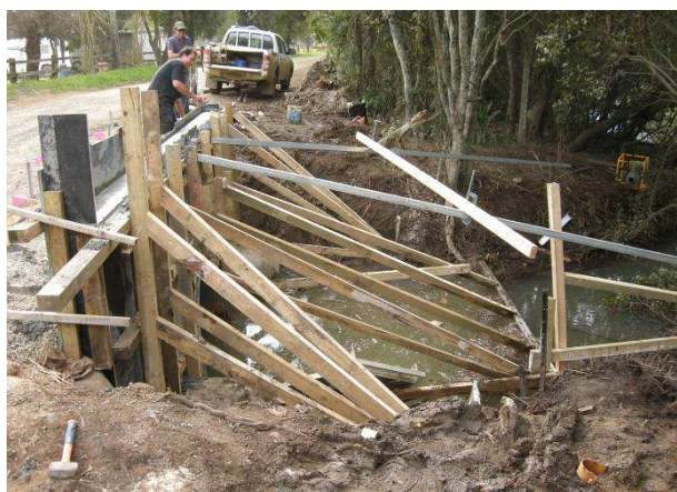
Image 65: cast in place concrete construction is intensive to both labour and cost
