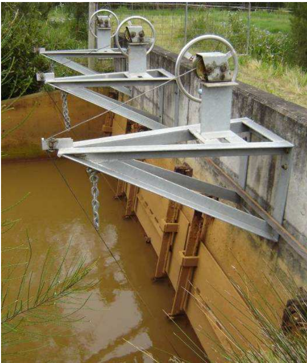
Image 19: winched flap gates on a horizontal lifting gantry (K Russell)
