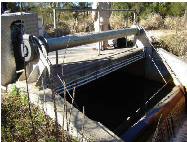
Image 53: single celled lay-flat gate in Partridge Creek, Port Macquarie
