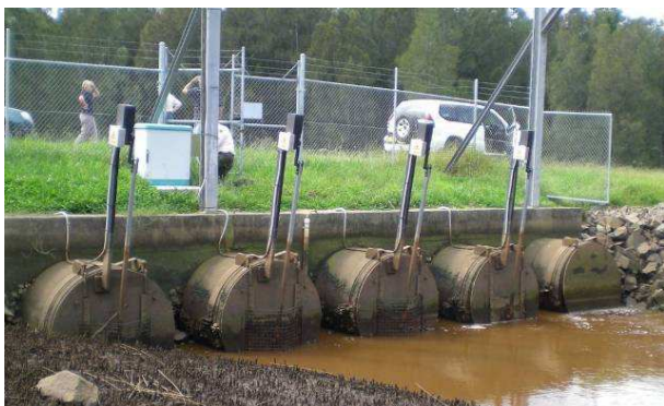
Image 35: smart gates installed in the Tomago Wetland (J Fredrickson)
