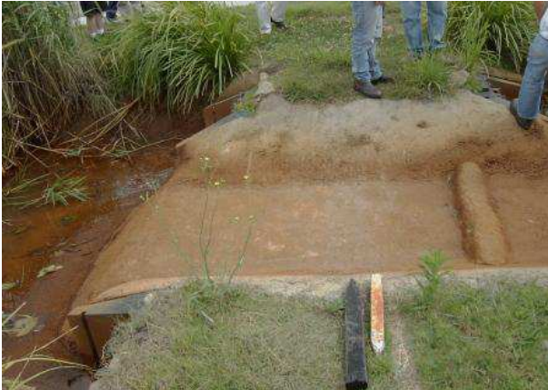
Image 43: permanent sill weir (Clarence Valley Council)
