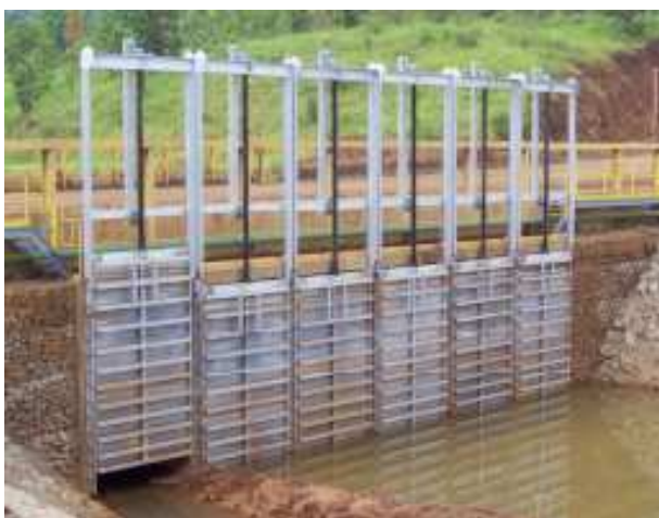
Image 23: multiple penstocks mounted on a gabion basket headwall (Watergates sp)
