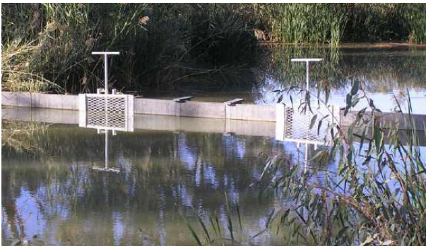
Image 38: solid plastic sheet piling weir with water control gates (Vonmac)
