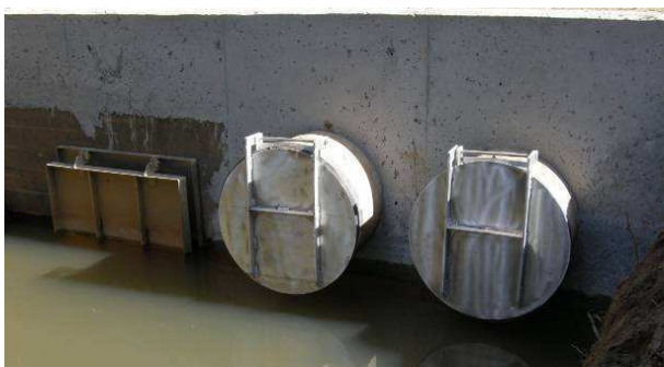
Image 9: top hinged flaps retrofitted to suit a box culvert and existing pipes
