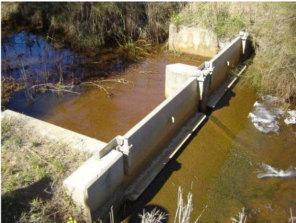
Image 44: concrete weir with flap gates for the prevention of saltwater intrusion. Compacted clay base covered by thin layer of concrete to reduce material costs.
