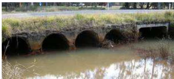
Image 4: Image combination of pipe and box culverts providing flow continuity under Port Stephens Drive
