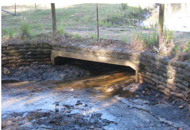
Image 8: sandbags can be filled with a concrete and sand mixture and stacked for cost effective headwall construction
