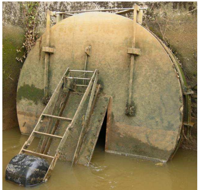
Image 31: automatic floodgate retrofitted to a pipe culvert at Windeyers Creek (J Fredrickson)
