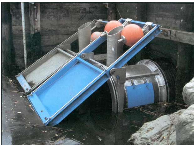
Plate 7: Automatic tide regulated floodgates
