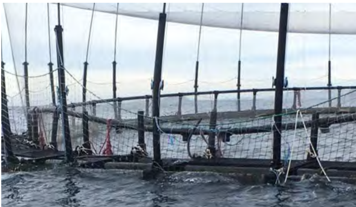
Figure 11: Picture showing dropped rail holding culture net which resulted from malfunctioned stanchion pins (Source: Huon, 2017).
