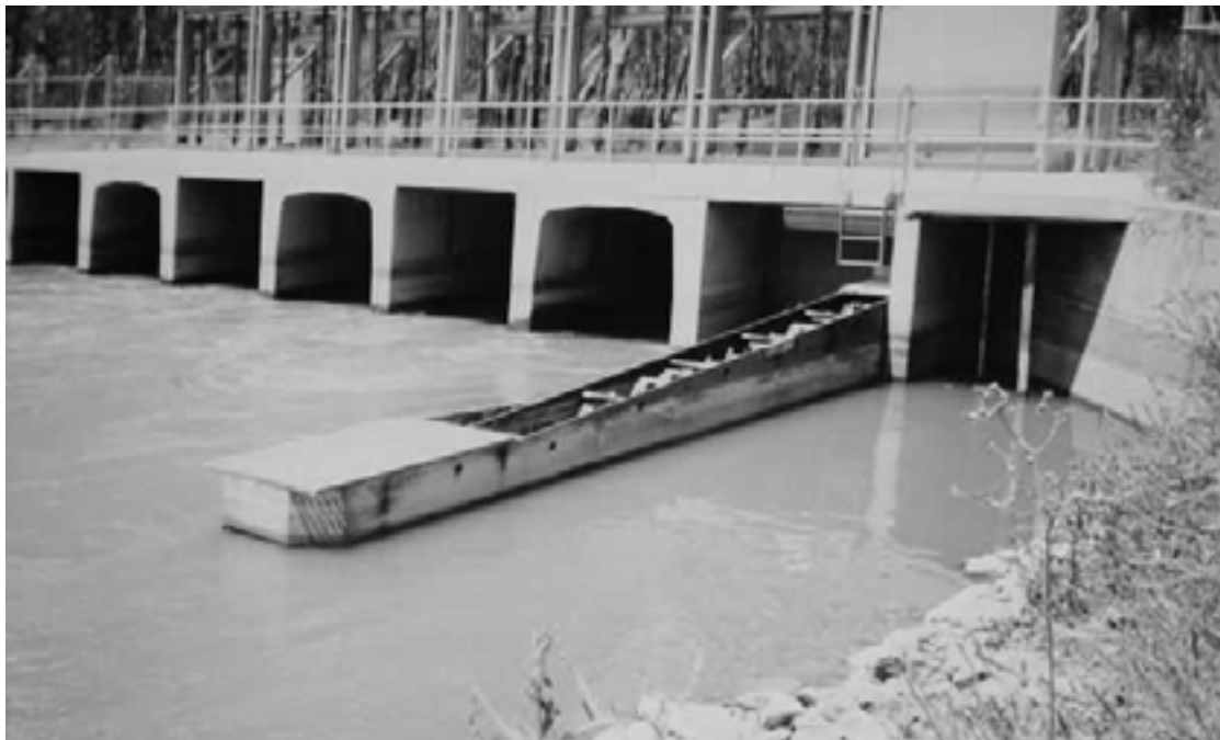
Figure 3. The Edward River Offtake regulator. The retrofitted Denil fishway is located at the right hand side of the structure.
