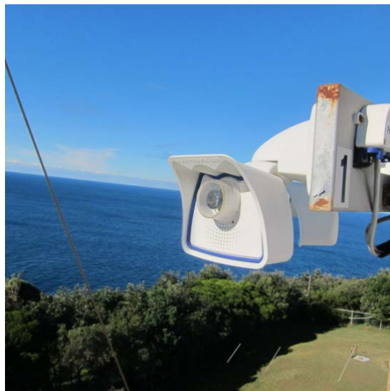
Figure 21 The motobox M24, 3 megapixel camera, mounted on the Old South Head Signal Station.
